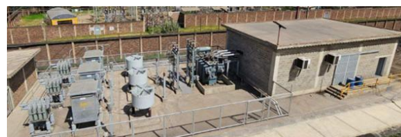
Figure 7 Photo of the Merus® STATCOM system on site.
