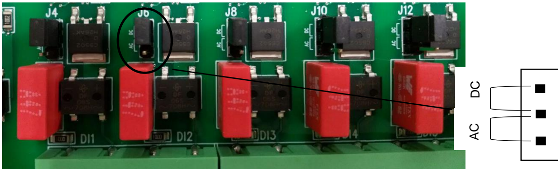
Figure 29: Input voltage choice on the AUX board, with one of the inputs magnified
